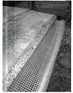
Quarter-inch welded wire mesh over gutters is first line of defense against rats crawling into this rainwater harvesting system. A water seal downstream stops mosquitoes.
