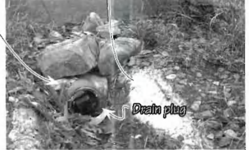
The completed drain was stoppered with a 4" plug (a cap would be better.) The concrete around the drain takes the pipe wrench torque from removing the plug, so the drain doesn't twist and tear out of the bottom of the tank.
