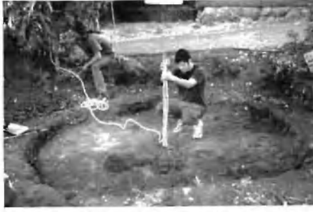
2. Grading the excavation with slope to the drain, using a water level.
