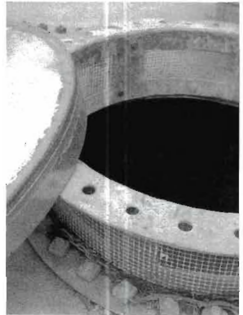
Critter-proof service access, air vent, and backup overflow all in one. Note that vents around access are screened with 1/4" hardware cloth over mosquito net.
