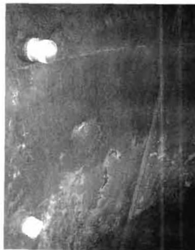
Giant sheets of rust peeling off the inside of an old galvanized bolted steel tank. Upper inlet has brass nipple in it; the lower inlet has a PVC male adapter. In each case the function is to keep the threads usable.
