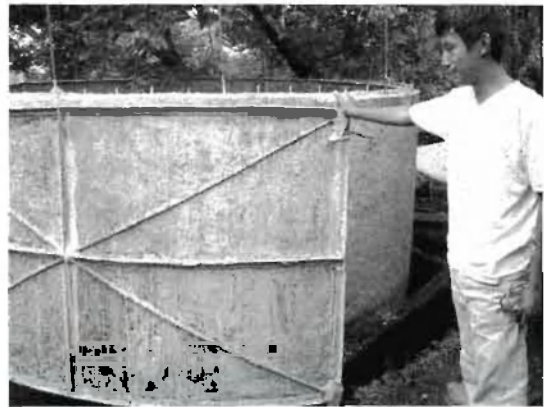
Pulling reusable steel forms off of a new concrete tank in a Mexican village.
