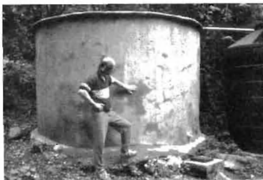
Here a 20 year old, ultra-light-duty ferrocement tank gets a re-plastering in an effort to slow its disintegration, with mixed results.
