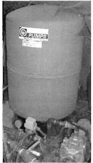
Pressure tank and pressure pump.
