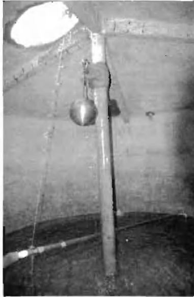
Same tank inside. A ladder could have been incorporated in the central pillar, for safety, and to avoid the hassle of feeding an extension ladder into the tank.
