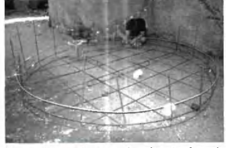
3. Bending and tying rebar for the floor (note—wall in background is ferrocement, too).
