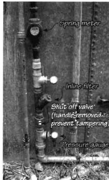
Inlet hardware. Pressure gauge before shutoff shows static pressure. Pressure gauge after shutoff shows dynamic pressure across filter, which shows when it needs service.
