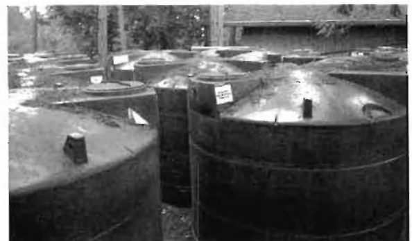
A tank farm for a rainwater harvesting system on San Juan Island, Washington State. The tanks are connected in series at the bottom, so they all rise and fall at the same level, and the water does not stagnate.
