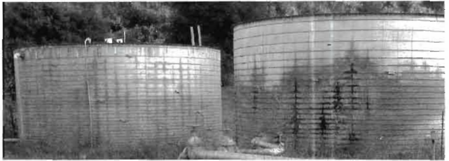
Two 70 year old redwood tanks, one leaking, one not. The water in this system is highly sulfurous and quickly corrodes galvanized tanks.
