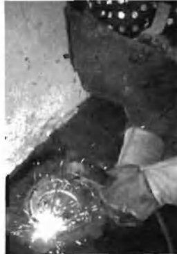
The whole assembly was then welded to the bottom of the old, assembled tank from the inside.
