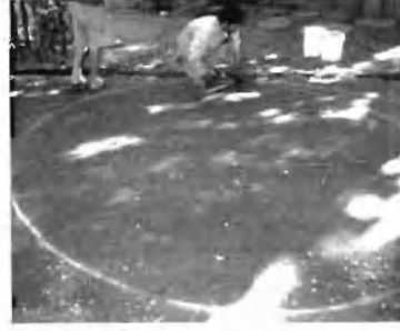
8. Circle drawn on driveway as guide for shape of horizontal rings of rebar.
