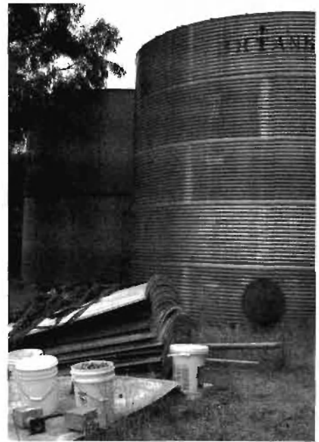
A good quality, 50+ year old bolted steel galvanized tank (with smooth surface, in background) and a less than 15 year old cheap, riveted galvanized steel tank (with corrugations, in foreground). Though much newer, the cheaper tank shows signs that it will fail before the older, higher quality tank. The pile of parts in the foreground is for another good quality, bolted galvanized steel tank.
