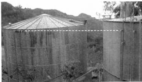
Connecting to a second tank with a maximum water level a foot lower resulted in the loss of 5,400 gal of useful capacity—thousands of dollars worth—in the first tank (at right), as the overflow had to be lowered to avoid having to duplicate all level-regulation hardware.
