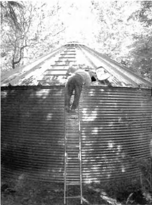
The access on this 50,000 gal (190 m 3 ) galvanized/poly bag tank is from the top only, as a perforation of this size of the liner would not be a good idea. Attempting to fill the 8,000 gal (30 m 3 ) or so of space under the lightweight conical roof with water would be equally inadvisable.
